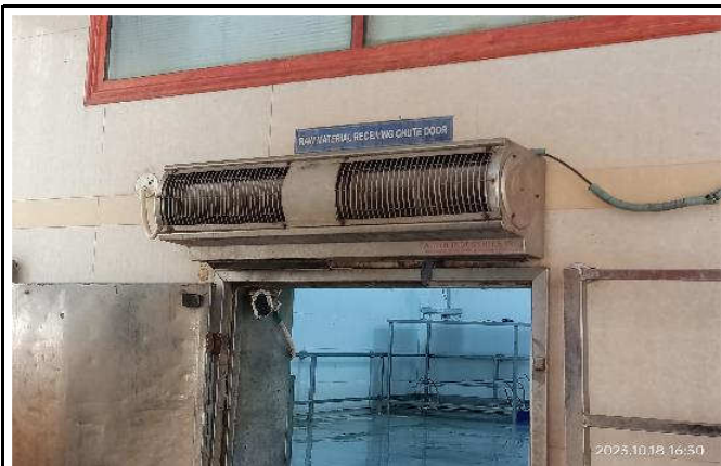
Raw Material Receiving Chute door air curtains need to be arrange to control the pest
