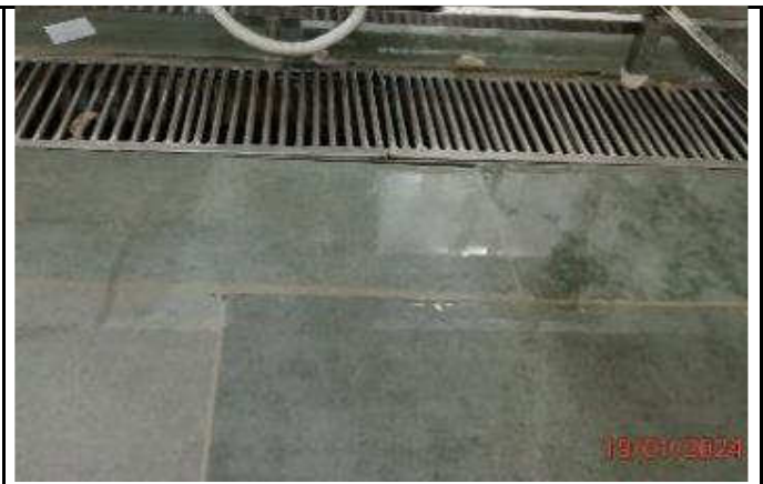
some pieces are found near by drain at soaking area.
