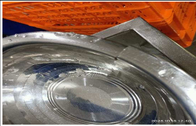
Damaged Steel Basins are observed.
