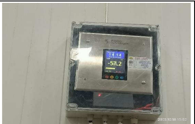
digital meter is working but not accurate
