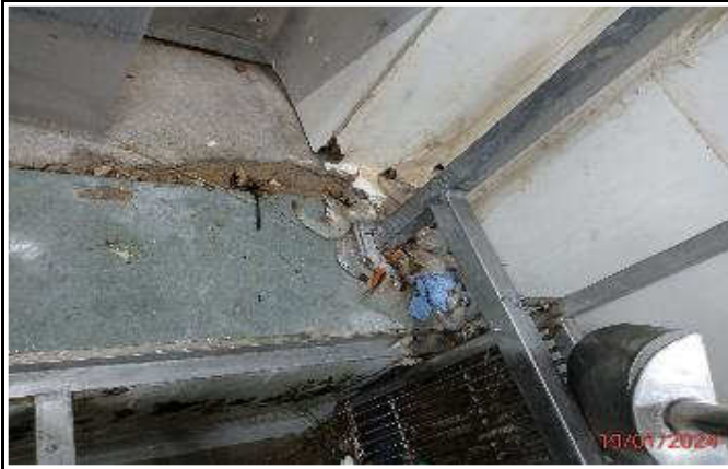
Some pieces are found near by drain at raw material receiving area.
