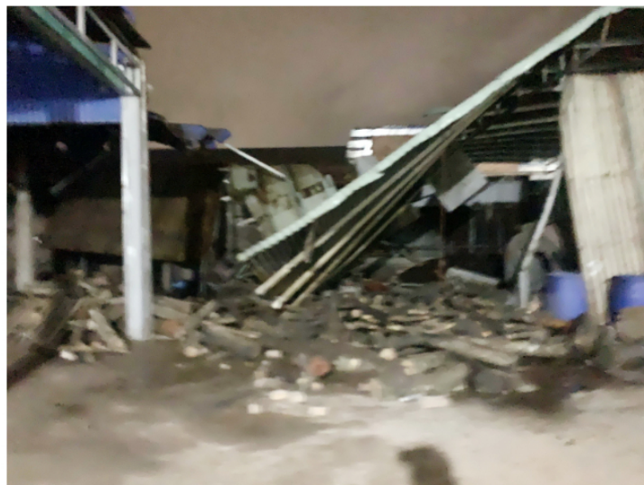
A section of the prefabricated factory roof collapsed after the explosion.
