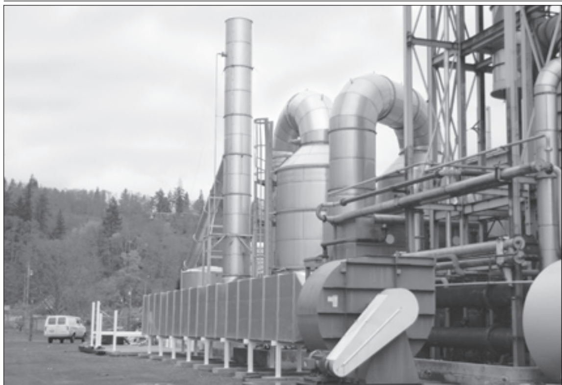
Ocean Protein’s towers scrub odorous compounds
