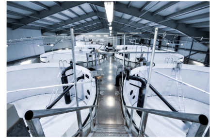
RAS tanks ready to be filled with water and fish. Photo: © Pure Salmon Technology.
